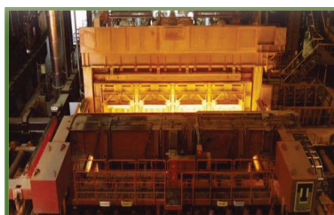
Walking Beam Furnace
